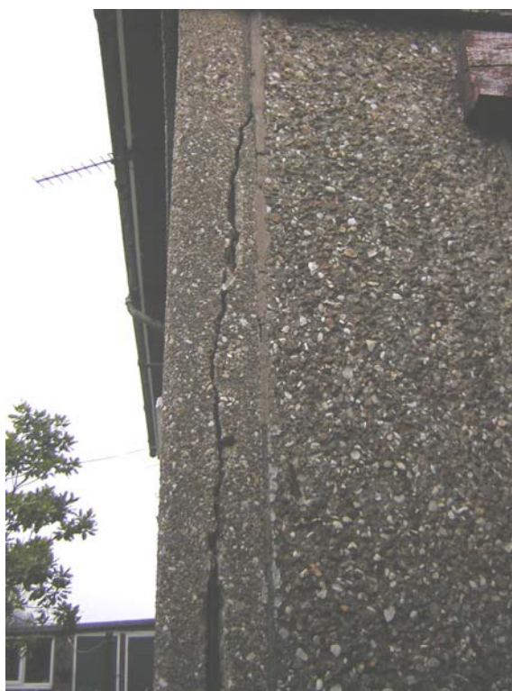
Photograph 2 – Vertical Cracking Of Corner Post
