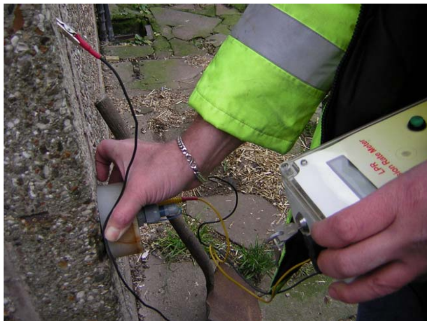
Photograph 4 – Linear Polarisation Corrosion Rate Monitoring
